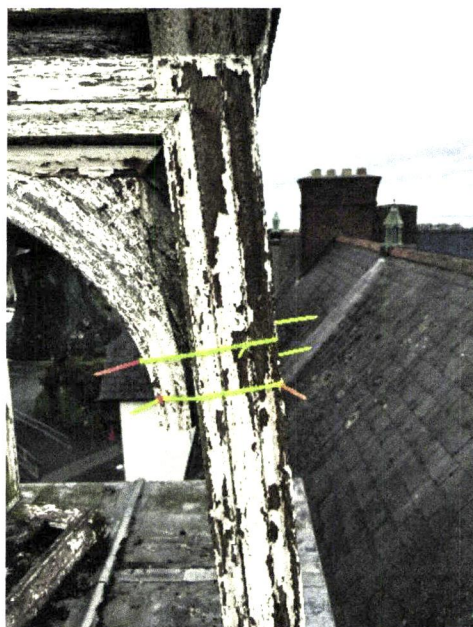
Photograph 16: Loose timber with temporary fixings to secure
