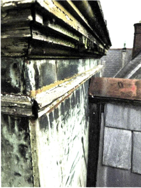
Photograph 21: Further view of dentil pieces missing and lower timber loose with nail failures
