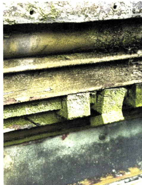
Photograph 20: Close up of timber dentil pieces with missing dentil pieces and one about to fail
