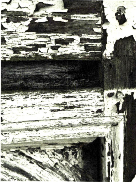
Photograph 13: Rot in decorative timber and structural horizontal member behind
