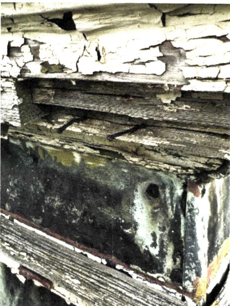
Photograph 15: Missing decorative timber and rot noticeable on timber behind
