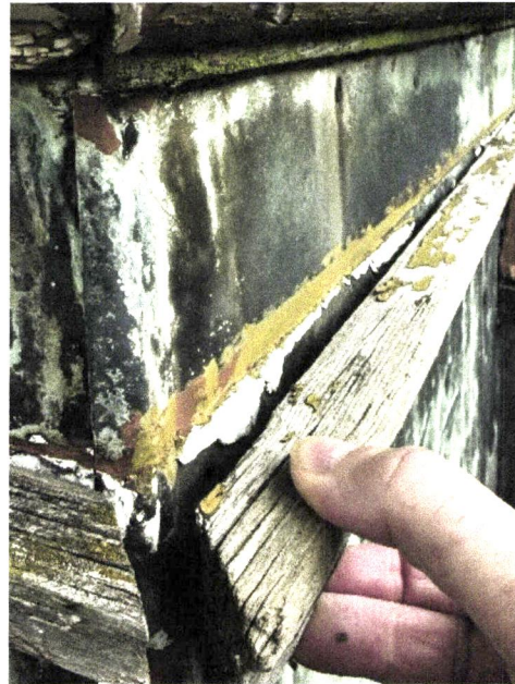
Photograph 14: Loose timber to copper shroud on dais support to bell tower
