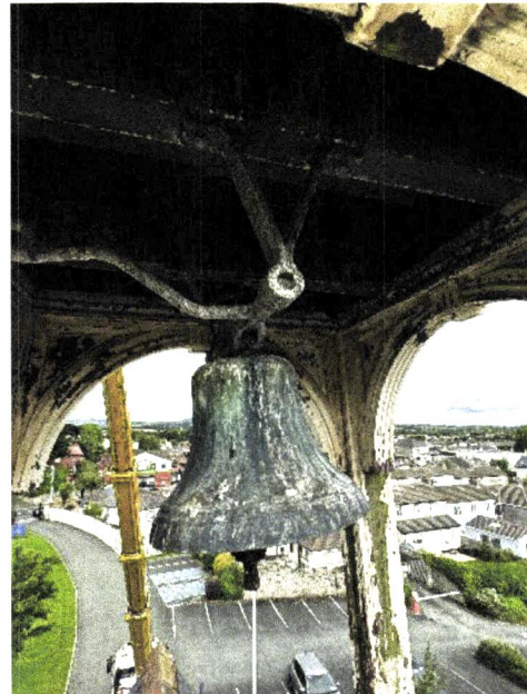
Photograph 4: View to underside of bell tower roof steel bell supports and timber cladding to ceiling
